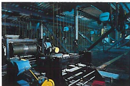
The power set-up in the roof, with a view across the over-stage grid.
